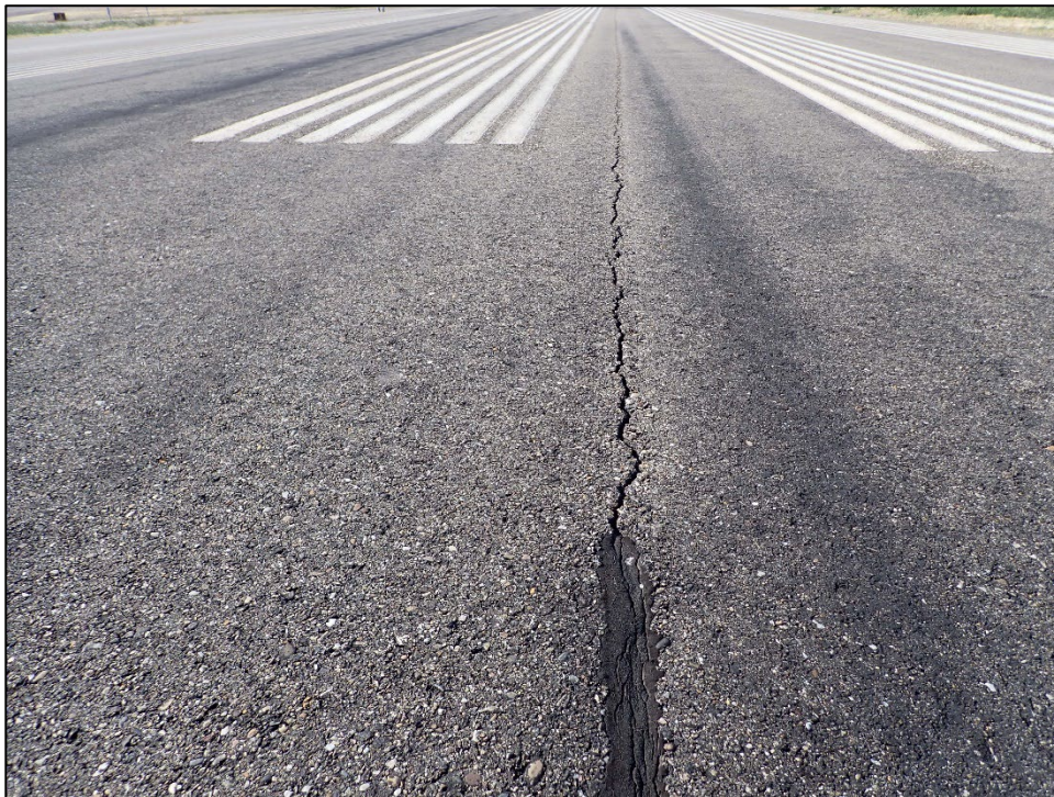
RW10-01-66: L&T Cracking
