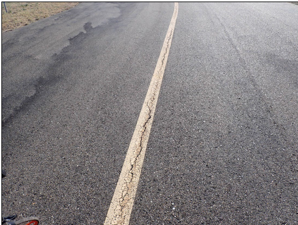
TW-01-07: L&T Cracking
