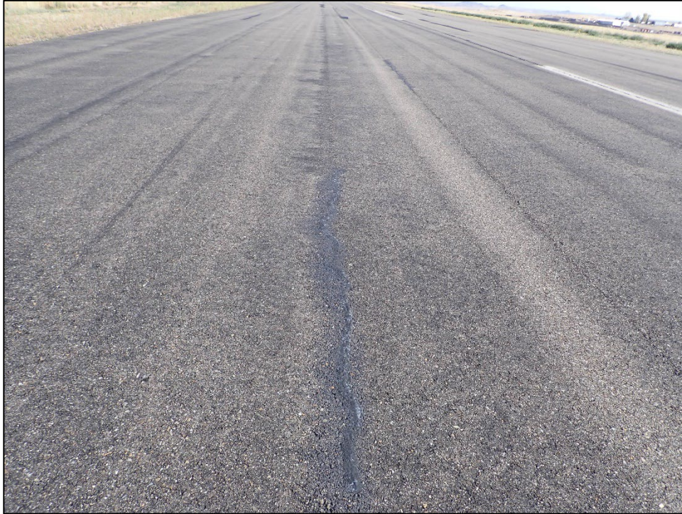
RW10-01-46: L&T Cracking
